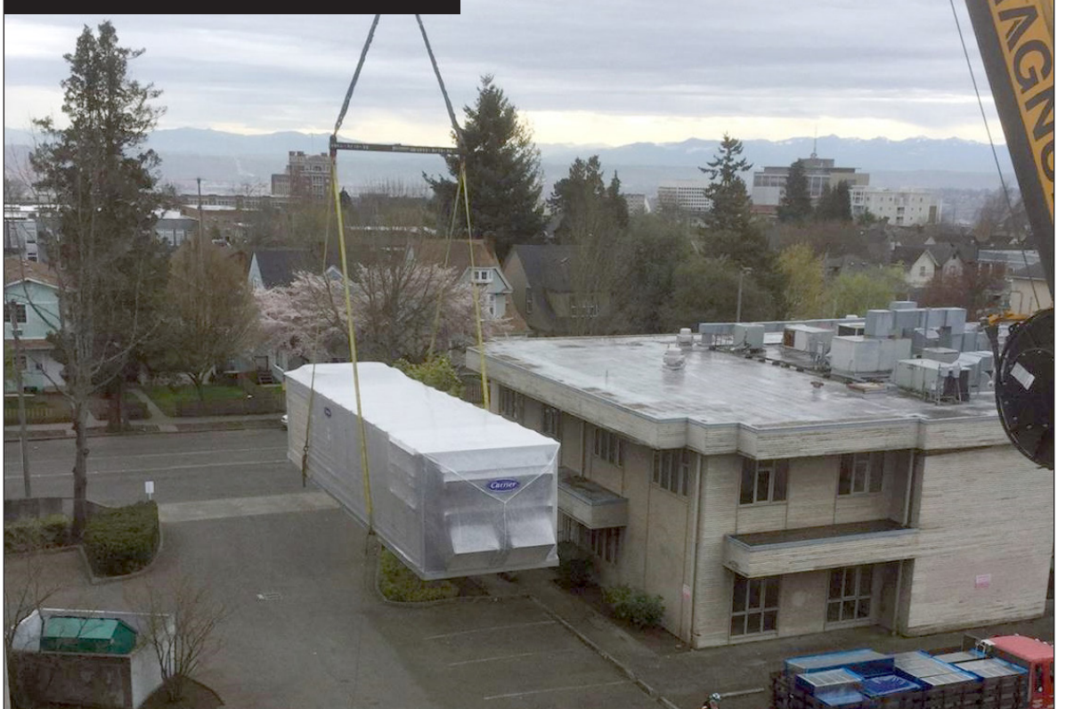
PHOTO FROM AIR SYSTEMS ENGINEERING
