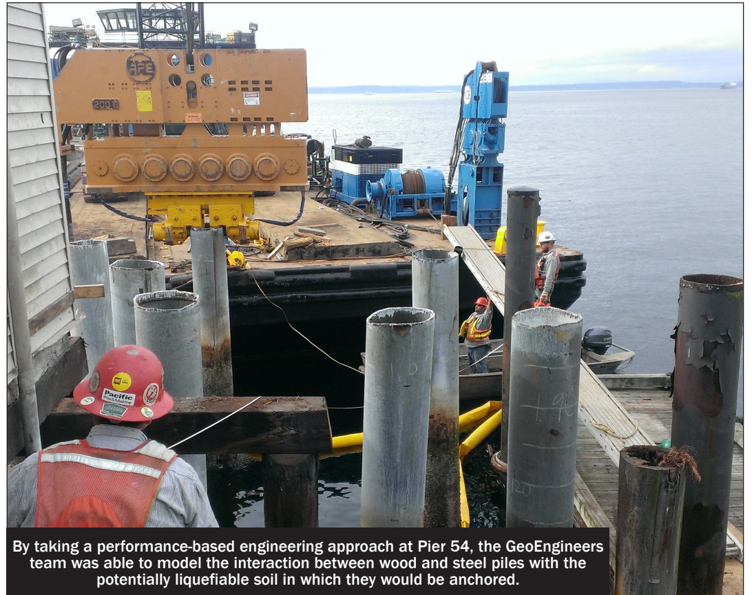
The seismic design recommendations for Ivar's Pier 54 improvements included the addition of steel pipe piles to reinforce the 100-year-old wooden structure.
