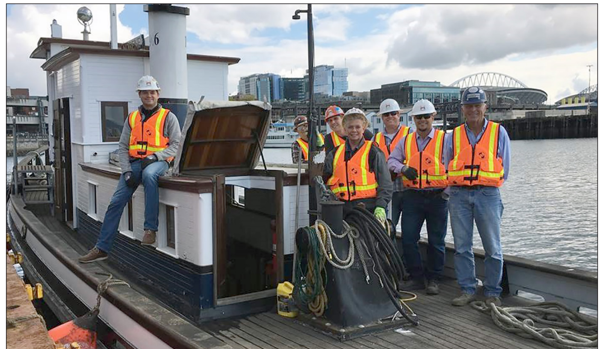
Part of the job involved working from the water side of the dock.
