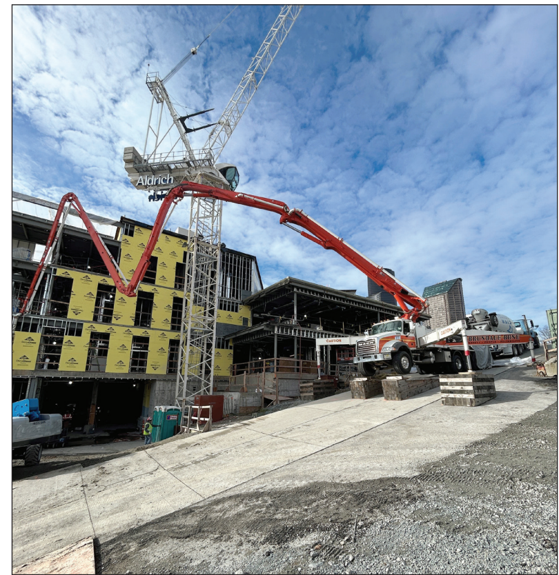
Superintendent Brett Price designed an interlocking ramp system to stabilize large trucks and cranes on the sloped site of the Northwest Kidney Centers' new flagship Seattle campus. Photo courtesy of Aldrich
