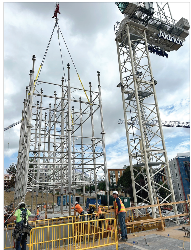
The NKC project required a 25-foot-tall shoring for a 14-inch concrete deck above. Instead of putting the forms together in place, the team preassembled the shoring poles in sections and craned each one precisely into place. Photo courtesy of Aldrich
