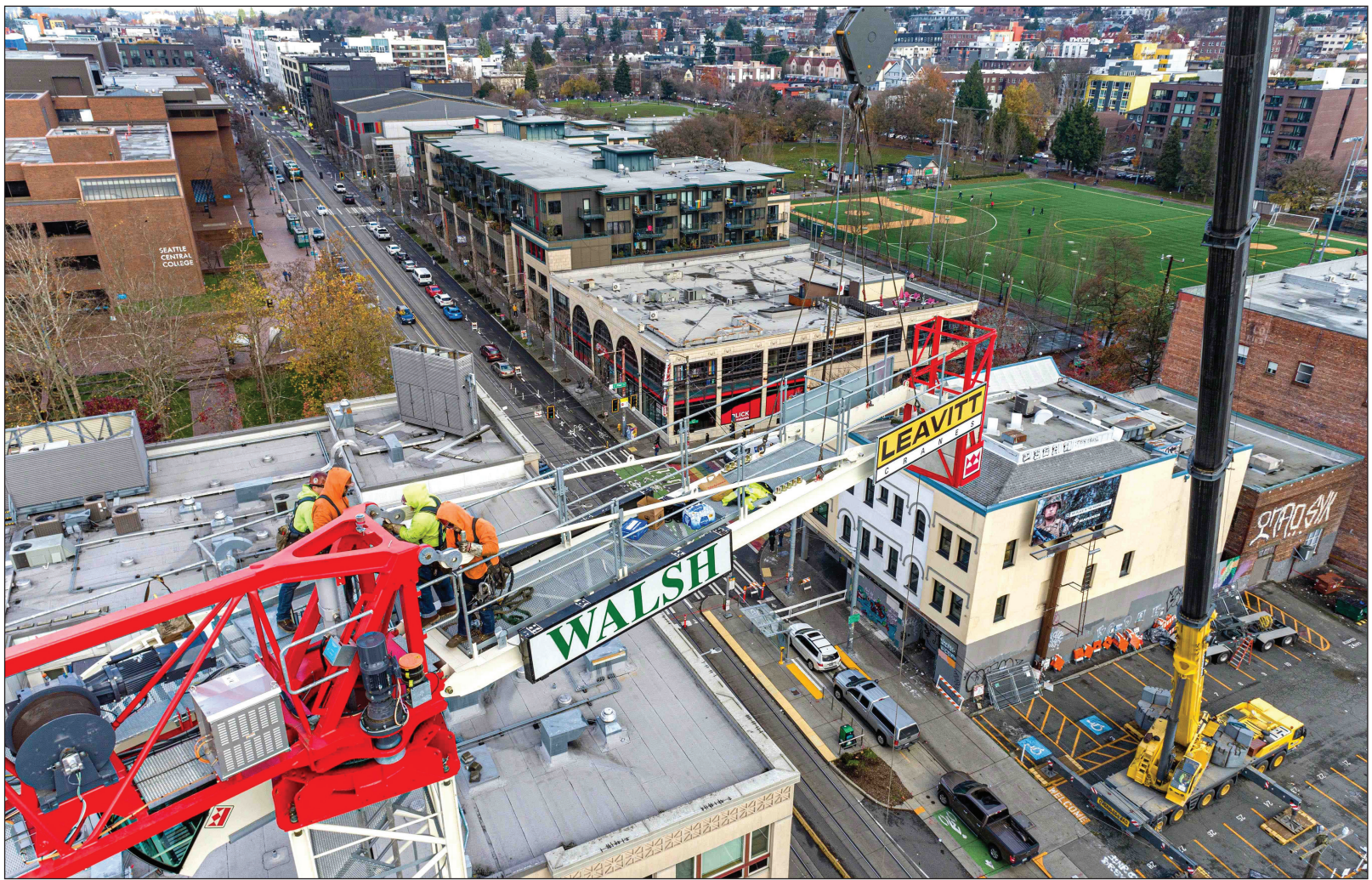
While the Walsh team installed and dismantled the tower crane at the Pride Place jobsite, all traffic was rerouted around that section of Broadway. Dozens of focused personnel were on site to safely manage each day. Photo by NW Skyview Imagery
