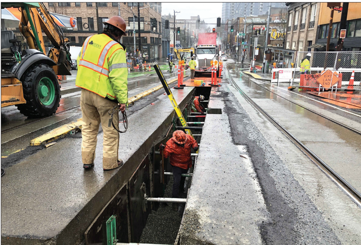
The project team was able to install water, sewer and storm connections safely and successfully, while maintaining bus and streetcar routes along Broadway, sometimes as frequently as every 3 minutes during peak commute times. Photo by Walsh Construction
